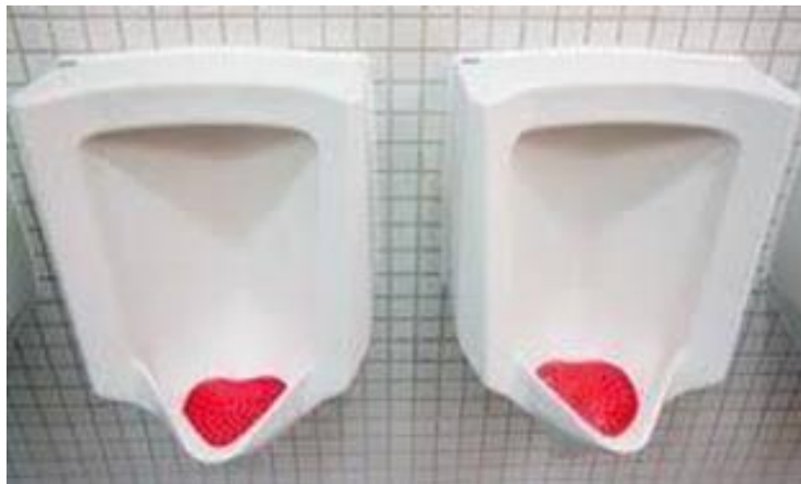
Figure 4-18: Water less urinals installed in the college
