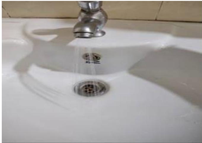
Figure 4-17: Low flow taps installed in the college
