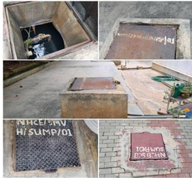
Figure 4-2: Sumps in the campus
