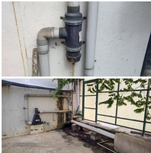
Figure 4-11: Rain water harvesting system in the campus
