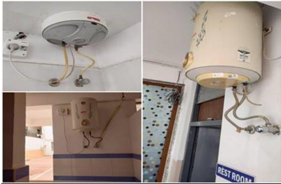
Figure 4-8: Electrical water heaters installed in hostels
