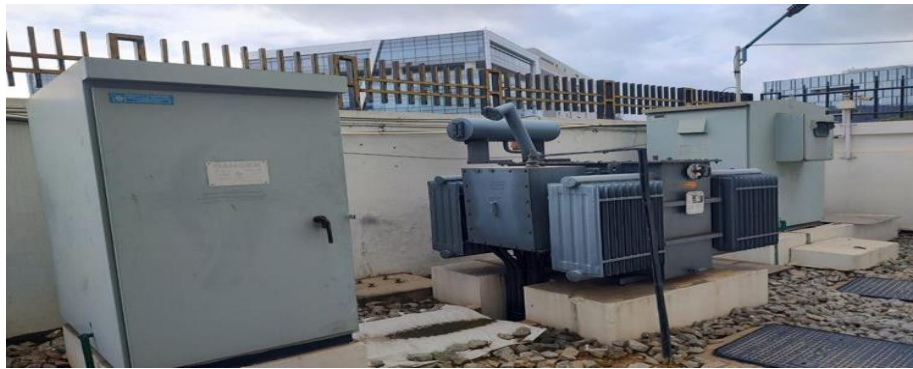
Figure 5-1: Transformer unit Installed in the campus
