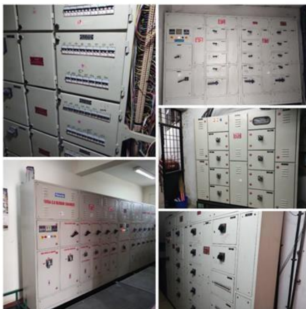
Figure 5-5: Electrical distribution panels in various blocks
