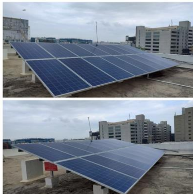
Figure 5-9: Solar rooftop PV system installed in NSB block
