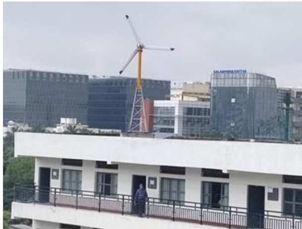
Figure 5-18: Micro wind mill installed in SVP block
