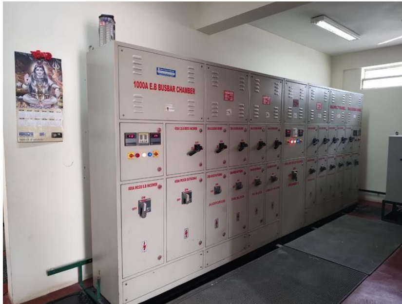
Figure 5-2: Electrical panel Room
