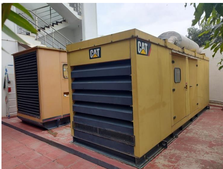
Figure 5-6: Diesel Generator (DG) sets
