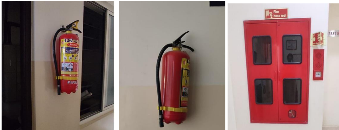
Figure 3-2: Fire Extinguisher and Fire hydrant system
