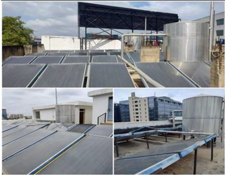
Figure 4-7: Solar water heater installed in the campus
