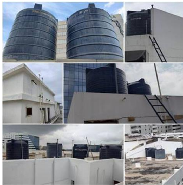
Figure 4-3: Overhead tanks in the campus
