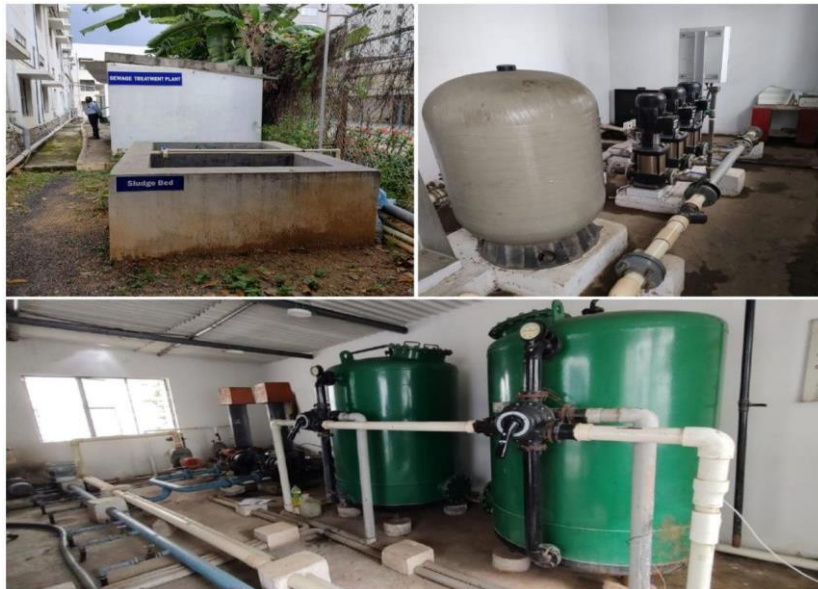
Figure 4-12: Sewage Treatment Plant
