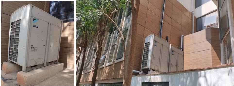
Figure 5-14: VRV Air Conditioning Unit
