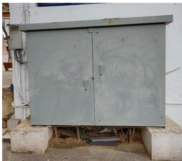
Figure 5-4: Feeder Pillar near NSB block
