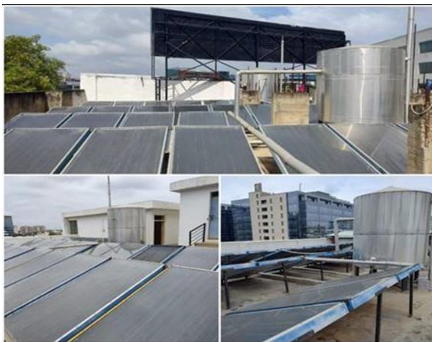
Figure 5-16: Use of Solar Water Heater
