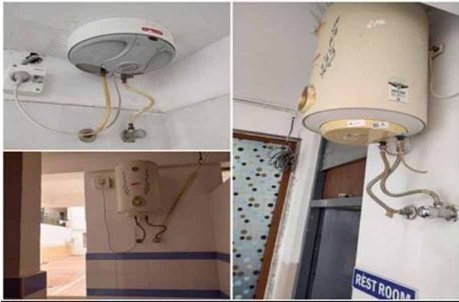
Figure 4-8: Electrical water heaters installed in hostels
