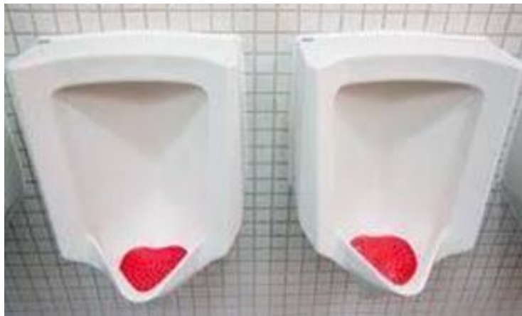
Figure 4-18: Water less urinals installed in the college
