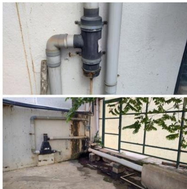
Figure 4-11: Rain water harvesting system in the campus
