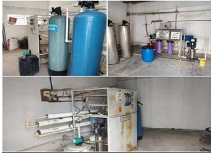
Figure 4-5: RO water treatment plant in the campus
