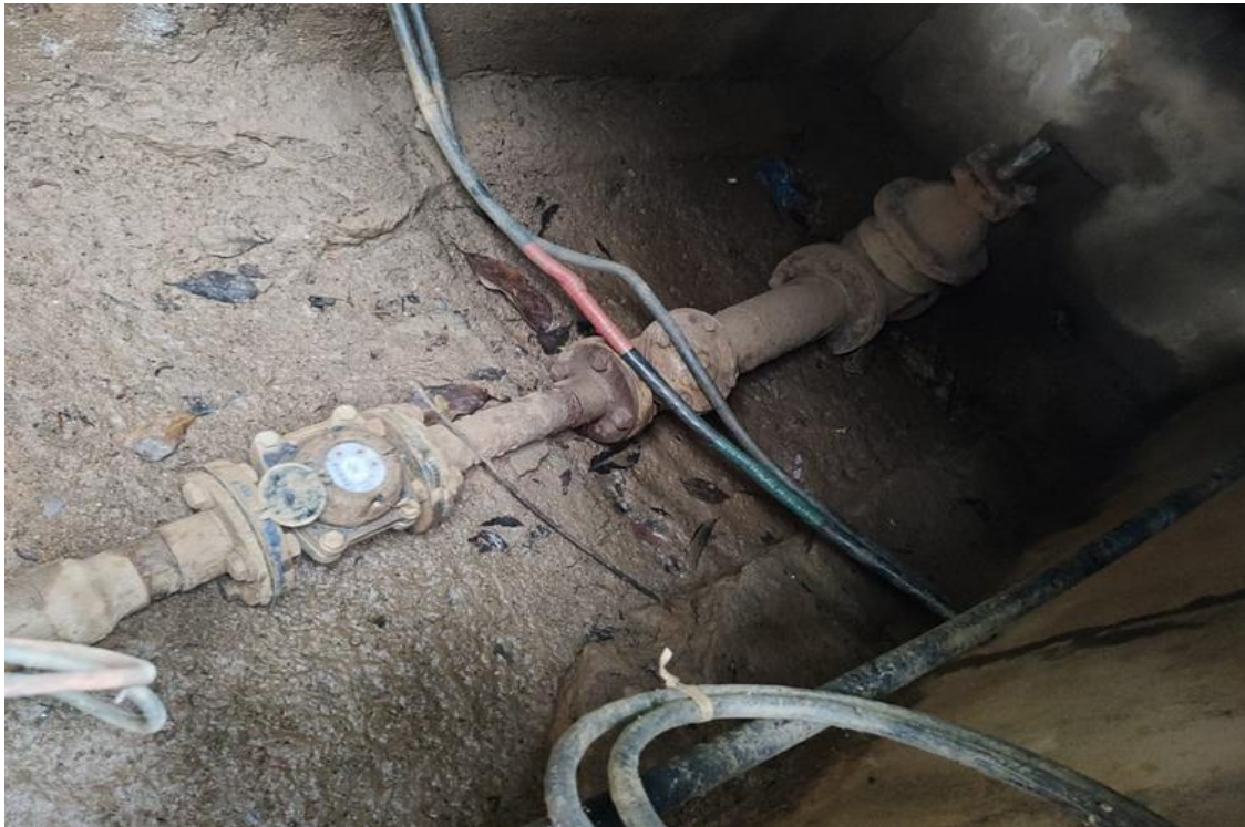
Figure 4-15: Water flow meter installed in the campus
