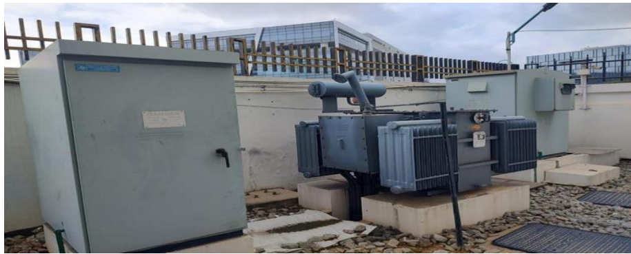
Figure 5-1: Transformer unit Installed in the campus
