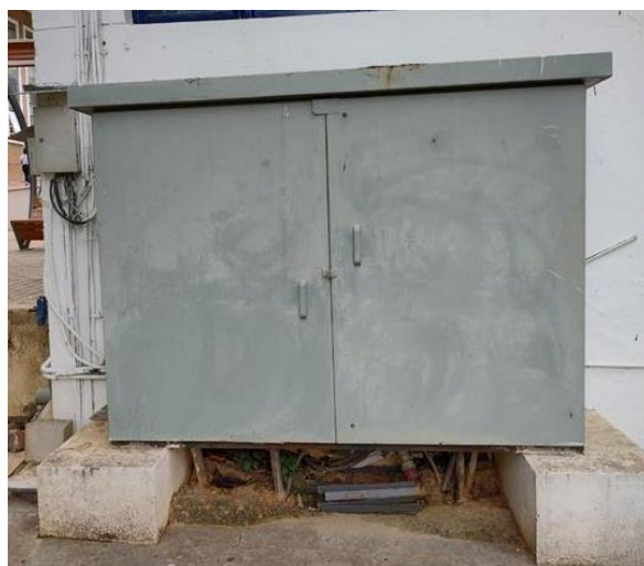
Figure 5-4: Feeder Pillar near NSB block
