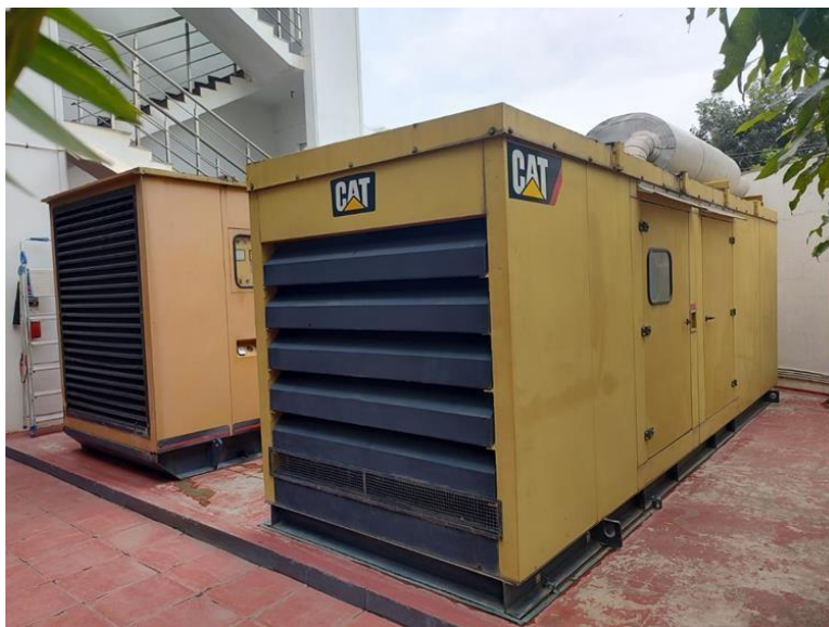
Figure 5-6: Diesel Generator (DG) sets
