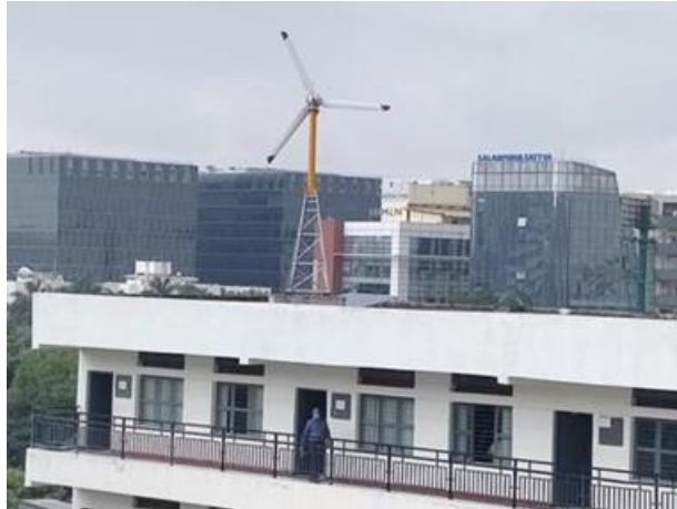
Figure 5-18: Micro wind mill installed in SVP block
