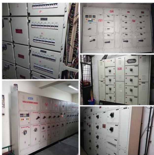
Figure 5-5: Electrical distribution panels in various blocks
