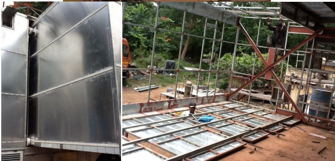
Figure 3a Major Guiding Wheels are partly seen at Top & Bottom (Left) and "X" Beams Fixed on eitherside (Right)
