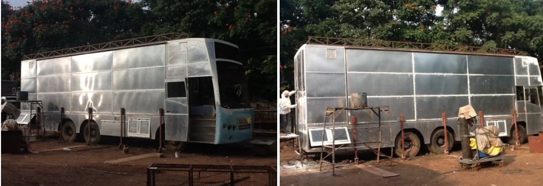
Figure 2 Five landing wheels which were assembled/attached to the outside body of expandable portion before the expansion
